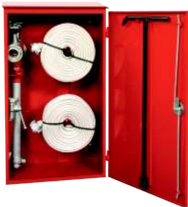
Hose and Equipment cabinet
